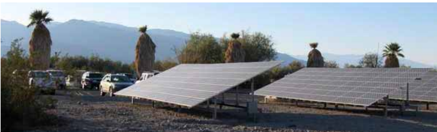
Furnace Creek Visitor Center solar panel system
